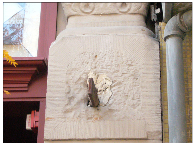
Careless placement of a sign can have lasting effects on the building.
